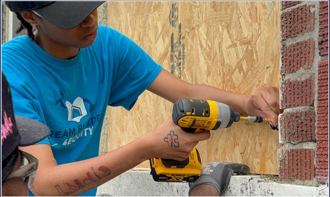
A volunteer works with Dream Builders 4 Equity to board up homes after the tornado.
